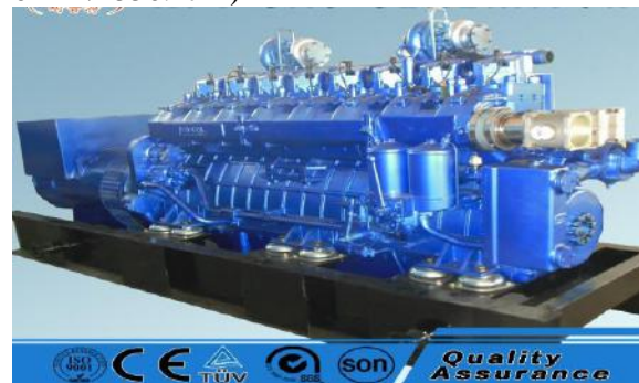
Gambar 6. Generator Biogas 325 Kw
